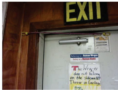
Exterior Door Does Not Close Properly
