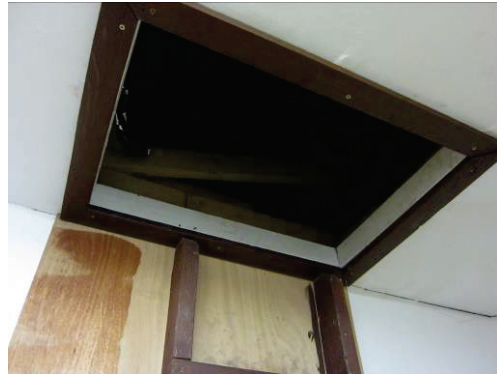
No Door Blocking Attic Draft
