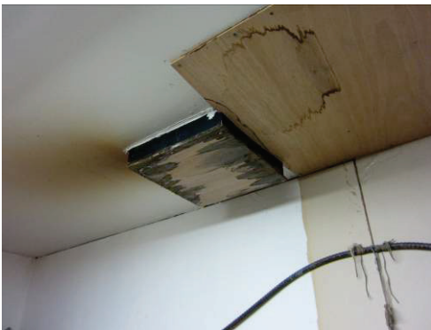
Blocked Furnace Exhaust and Burned Ceiling
