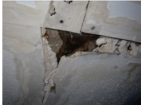
Ceiling Damage in Jailhouse
