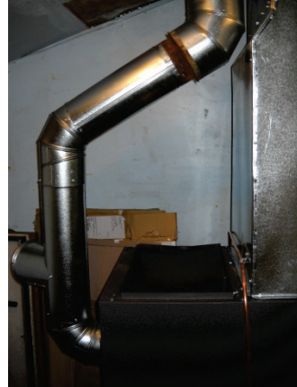
New Furnace and Stack
