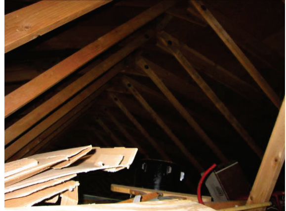
Not Much Insulation in Attic
