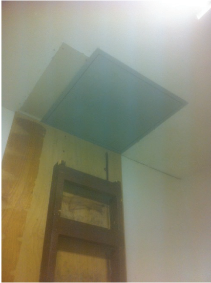
New Attic Access Door
