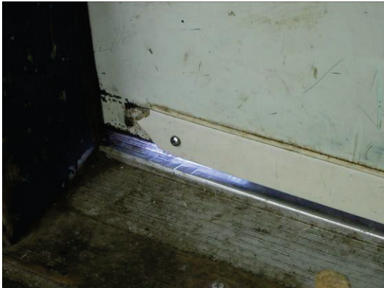
Doors Need New Weatherstripping
