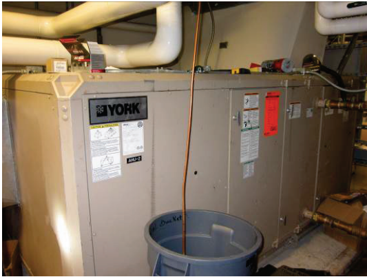
AHU-2 – York AHU
